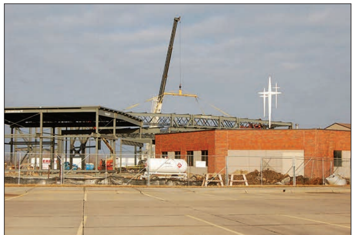
Construction of The Evangelical Free Church in Kearney, NE, financed by CIF
